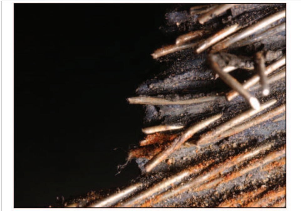
Figure 15.22: Broken steel cords of a stabilizer (steel belt) ply
